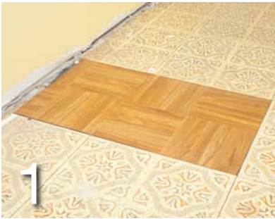
1 Repair or fill in low areas such as this spot where a built-in cabinet was removed.
