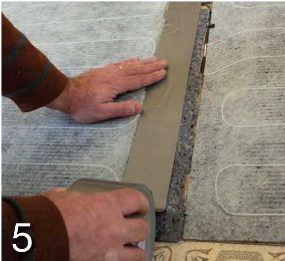
5 Secure the heat-mat ends, underlayment and wires to the subfloor with duct tape.
